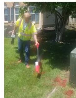
Bill Moore, utility locator for NOVEC, marks where current underground power cable is located.
