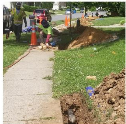
The "ground missile" (foreground) emerges after it has laid the underground pathway for new power cable along Parcher Ave.
